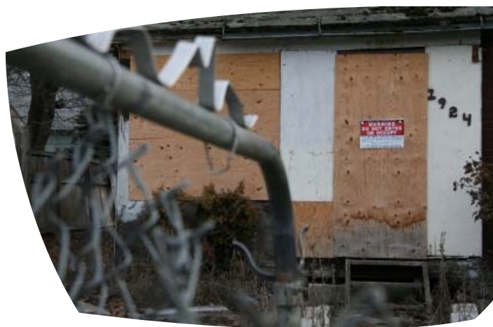
The processing of cooking methamphetamine can create so much damage that a structure is uninhabitable
