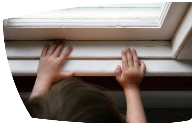
Lead paint can easily be inadvertently ingested by an unsuspecting child.
